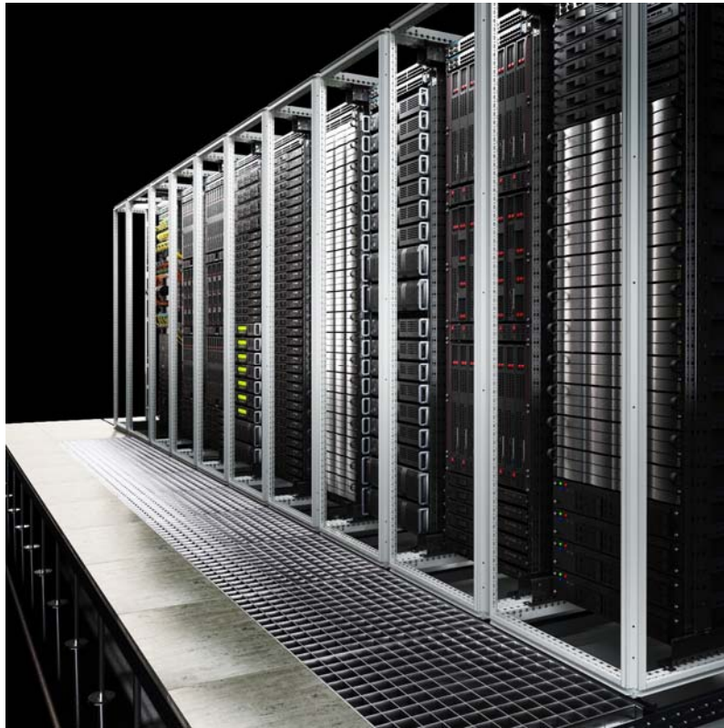
Figure 4: Example of a server module
